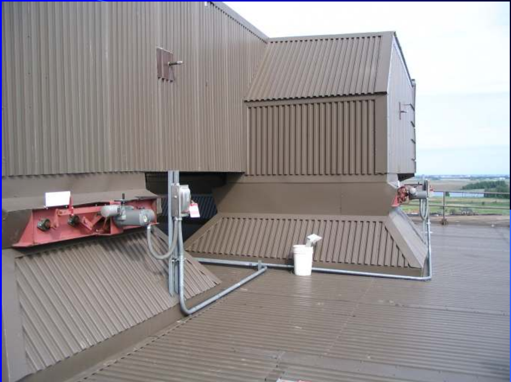
Outlet Plenum Vaned Dampers
