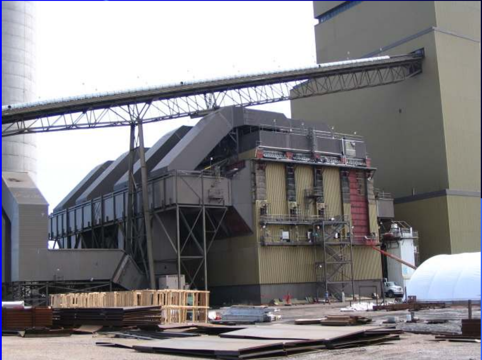
Big Stone Unit 1, Four Parallel ESP Chambers
