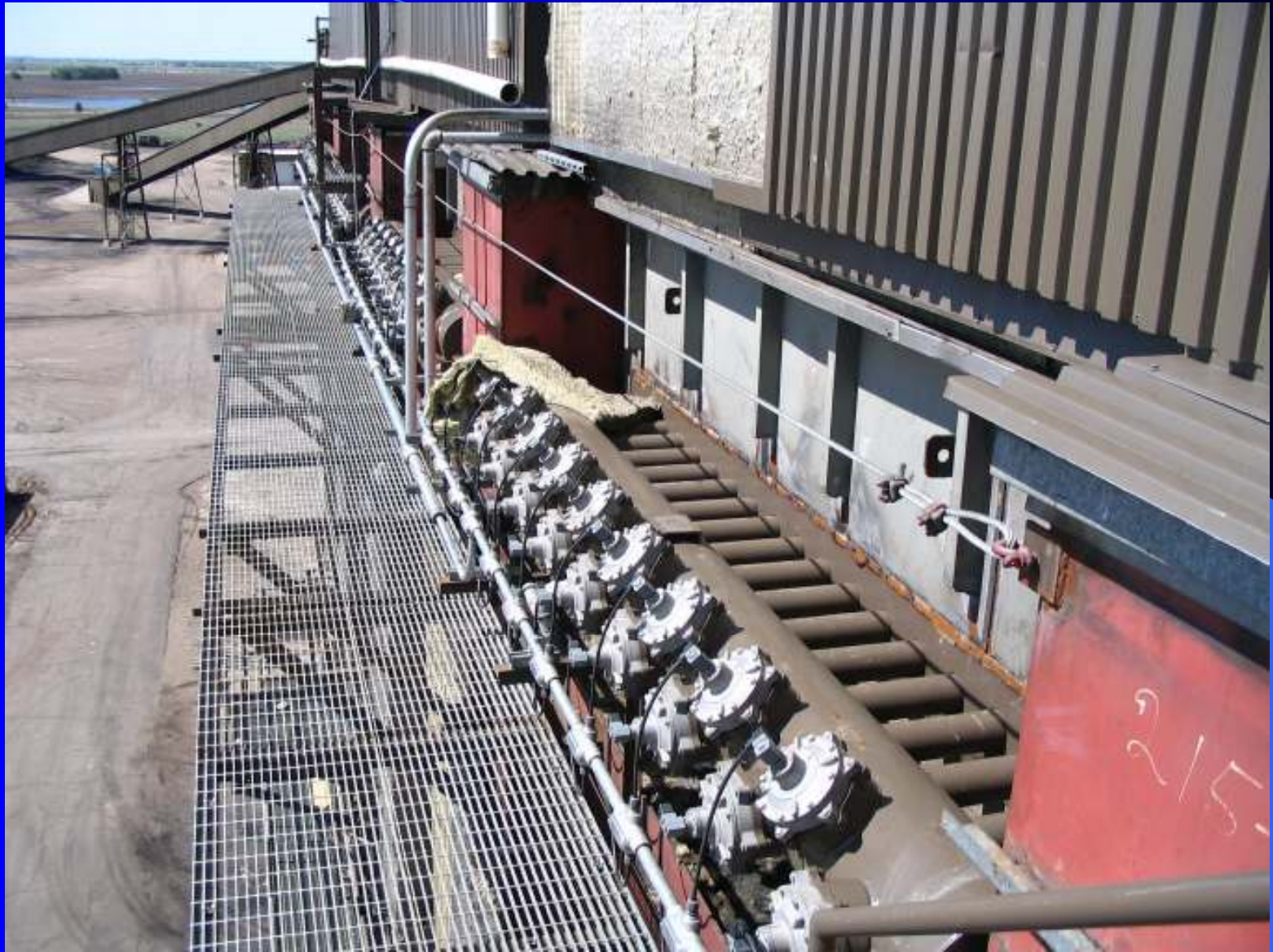
Pulse Headers – 4" Valves
