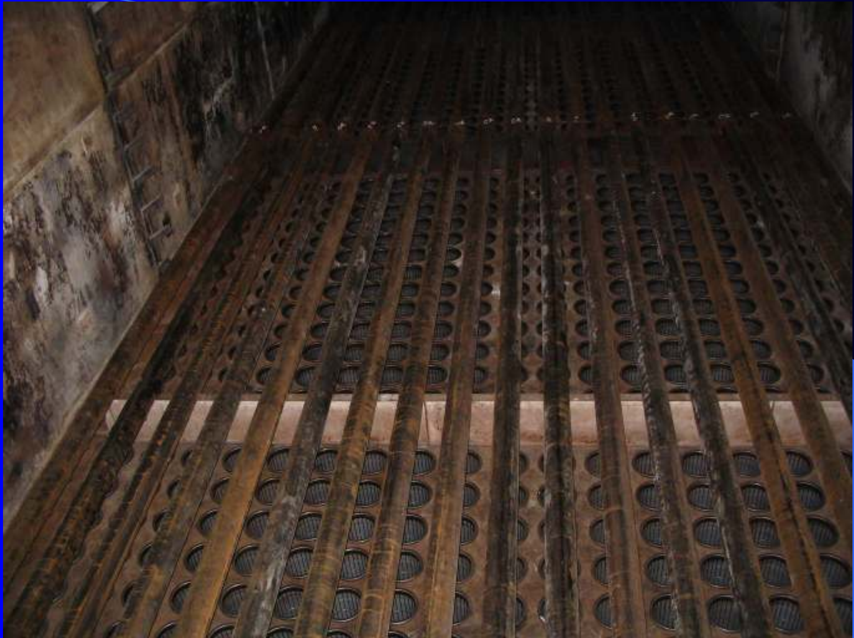
One Compartment's Tubesheet
