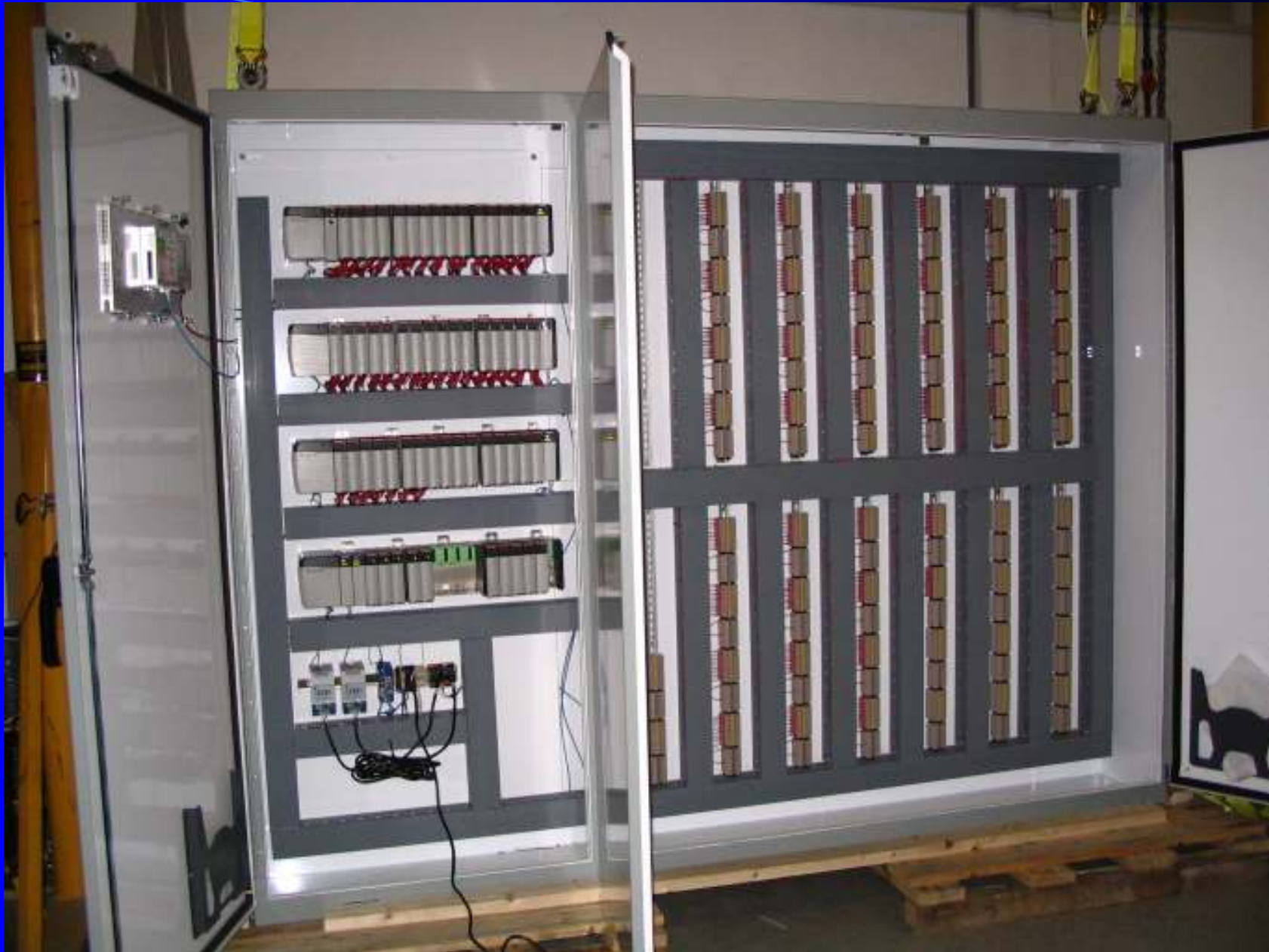
Allen Bradley Logix 500 Control Cabinet
